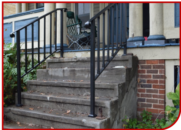
Figure 94: Example of an inappropriate railing replacement on a residential building.
