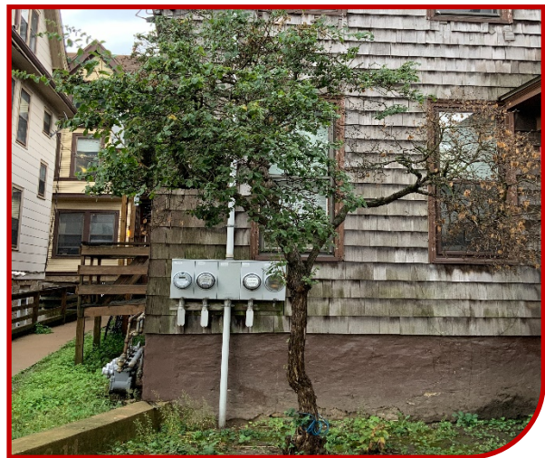
Figure 74: Example of inappropriately located utilities on the front of a historic residential building.
