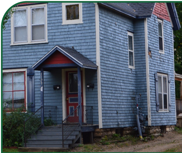
Figure 73: Example of appropriately located and painted utilities on historic residential building.
