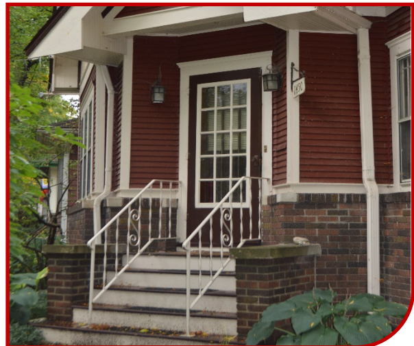
Figure 38: Example of inappropriate railings on residential building.
