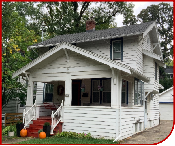
Figure 106: Example of inappropriate siding on residential building.
