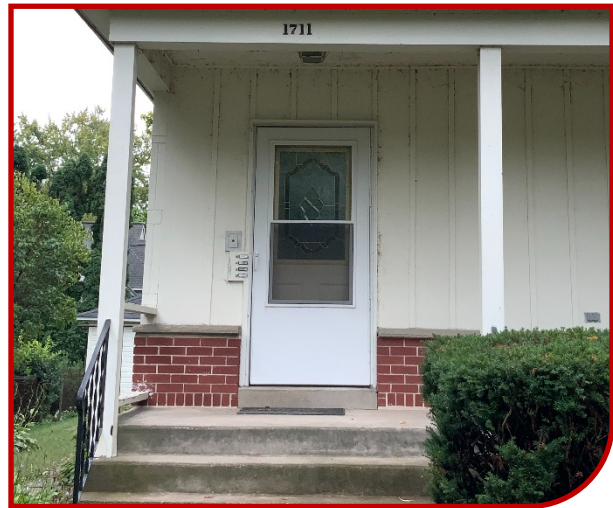
Figure 101: Example of inappropriate door on new residential construction.
