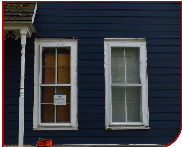
Figure 45: Example of an inappropriate modern window replacement that does not fit within the original wood casing on a historic residential building.
