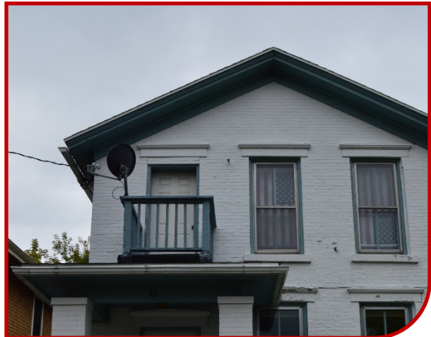
Figure 123: Inappropriately located satellite dish on residential structure.
