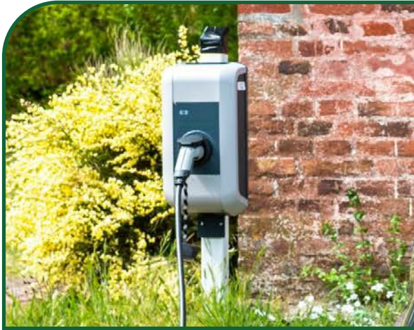
Figure 124: Appropriately located wall freestanding EV charging station at side of residence.
