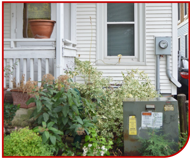
Figure 120: Example of inappropriate front location of utility installations on residential structure.
