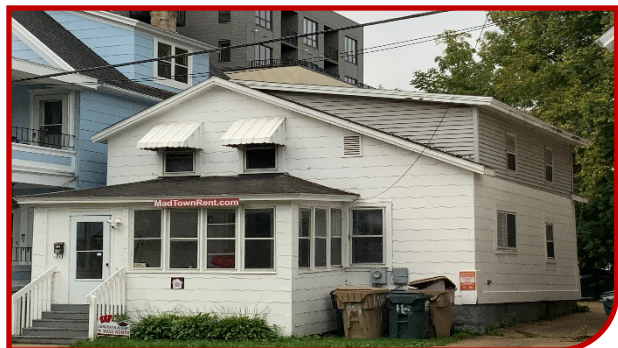
Figure 53: Example of inappropriate dormer addition to side of residential building.
