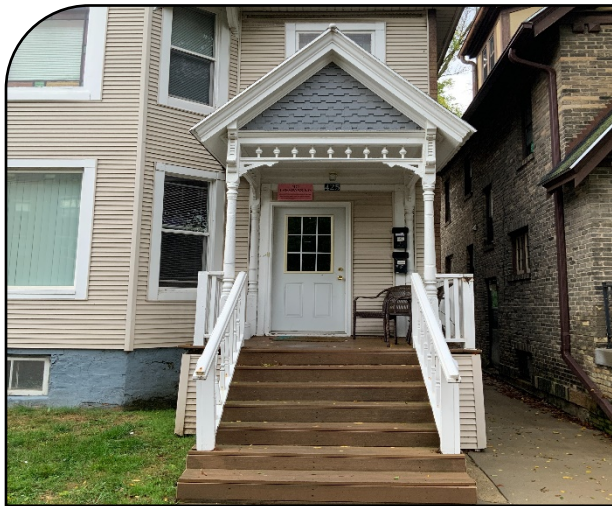
Figure 33: Porch flooring and steps replaced with compatible substitute material similar in visual qualities.
