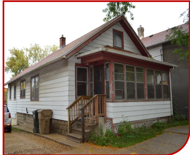
Figure 63: Example of inappropriately enclosed front porch on residential building.
