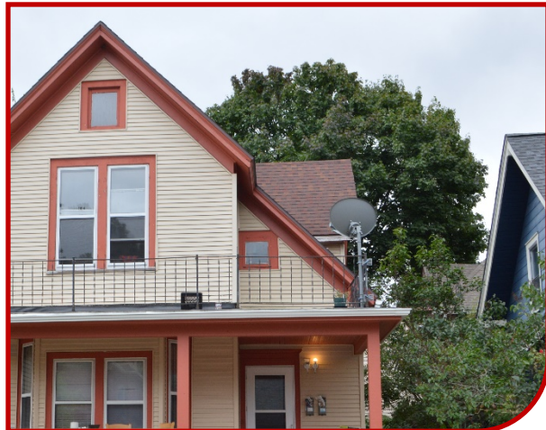
Figure 77: Inappropriately located satellite dish on front of residential structure.
