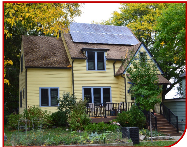
Figure 87: Example of inappropriate location of solar panels on front gable roof.
