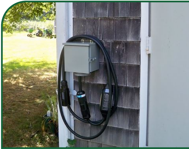
Figure 78: Appropriate residential wall mounted EV charging station.
