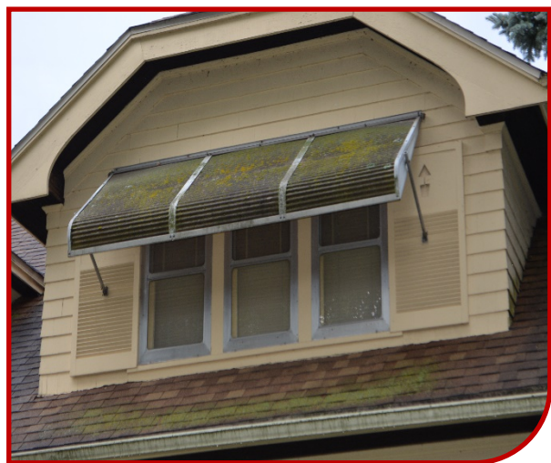
Figure 57: Example of inappropriate metal awning over shutters.
