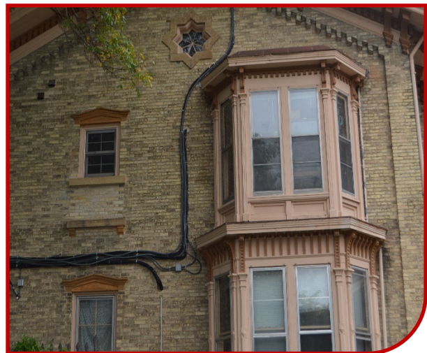
Figure 94: Example of inappropriately attached utility installations on a non-residential structure.
