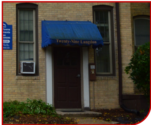
Figure 80: Example of inappropriate commercial door.
