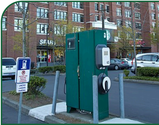
Figure 60: Appropriately designed freestanding EV charging station within commercial parking lot.
