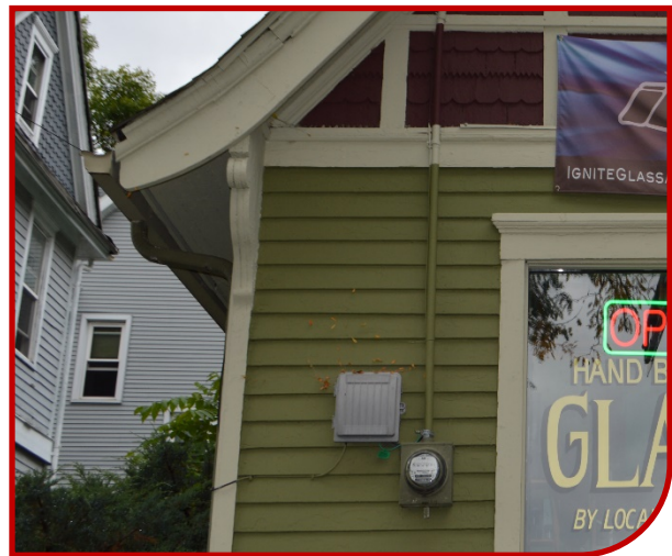
Figure 57: Example of an inappropriately placed and unpainted utility installations on a historic non-residential structure.
