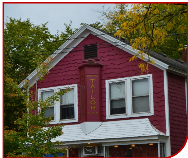
Figure 82: Example of inappropriate new siding on commercial building.
