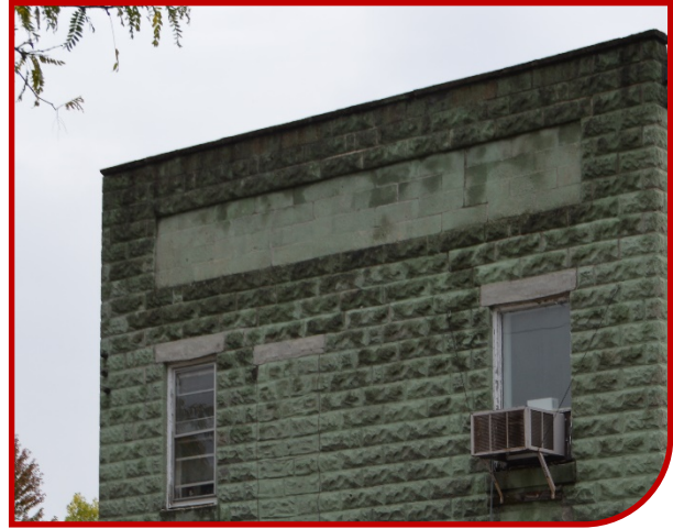
Figure 96: Example of inappropriate front AC installation on a commercial structure.
