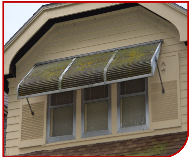
Figure 48: Example of inappropriate metal awning over shutters.
