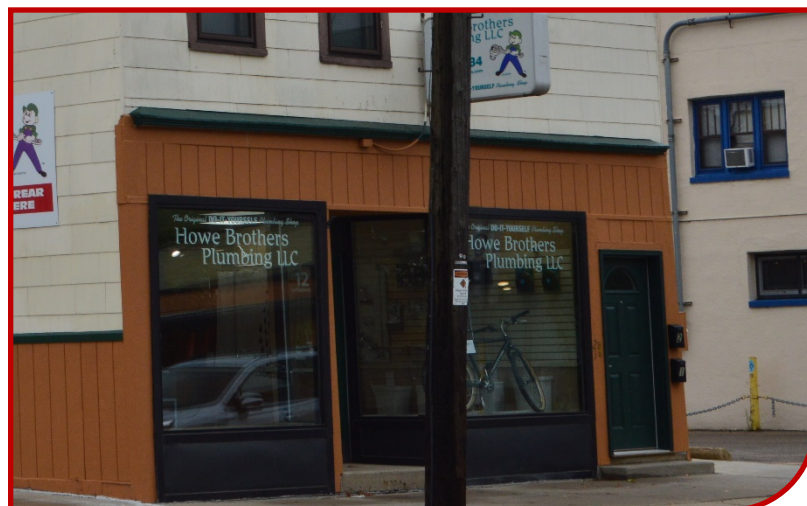
Figure 55: Example of inappropriate modified historic commercial storefront.
