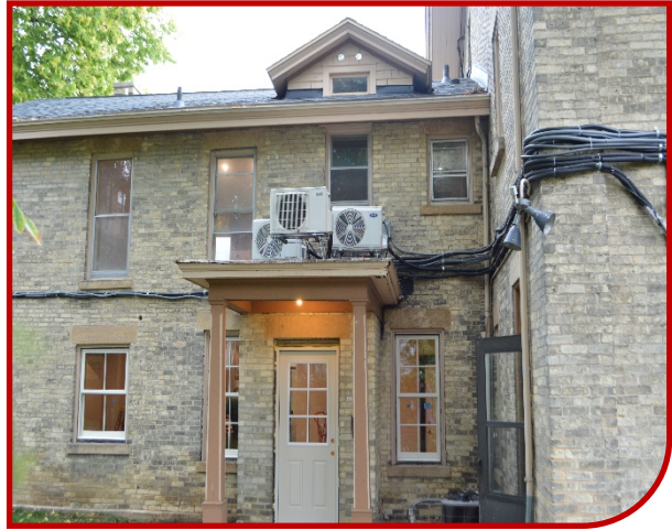
Figure 59: Example of inappropriately placed HVAC equipment on a historic non-residential structure.
