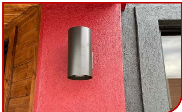
Figure 90: Example of inappropriate lighting on a commercial building.
