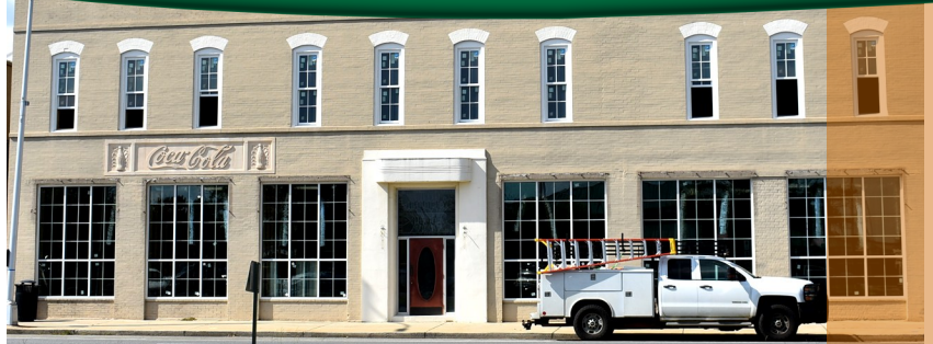
The old Ashley Place is undergoing major renovations. The building will become the new home for RW Griffin Executive Offices.
