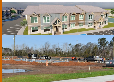
Sitework continues for the Platform Douglas housing development on Lupo Lane. -126 Units -Estimated completion in 2026.
