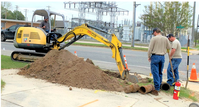
Douglas Natural Gas Technicians, Jake Phillips, Joey Casteloes, and Trace Tatum conduct maintenance on a natural gas valve located at the CE Weir Center. Markings on the ground help identify underground utilities and a fire extinguisher is near in case of an unexpected emergency.
